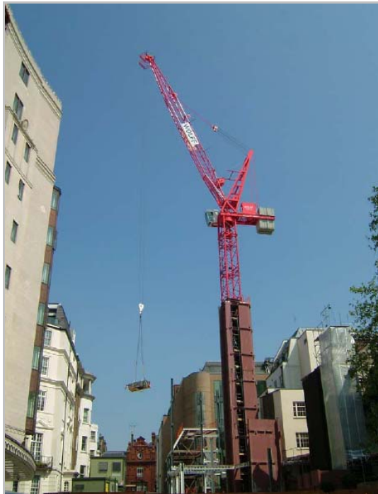
A tower crane was bolted to the top of a completed core to lift the remaining steelwork into place
