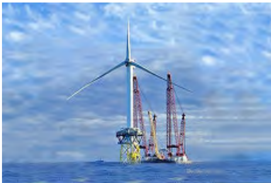
Steel plate for the pioneering Talisman Beatrice wind farm off east coast of Scotland
